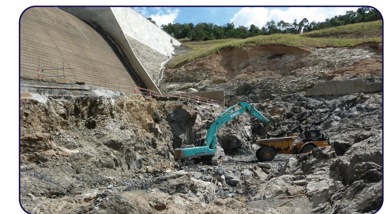
Downstream damage - February 2013
